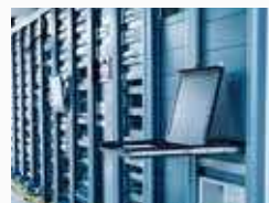
Control Room/ Data Center
